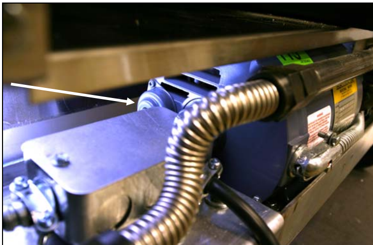
Filter Pump Reset Switch (Arrow)
